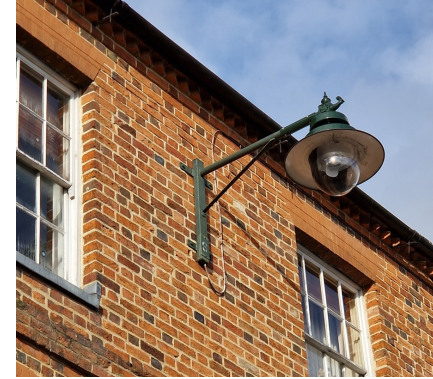
Wall streetlights in the Buckingham Conservation Area
