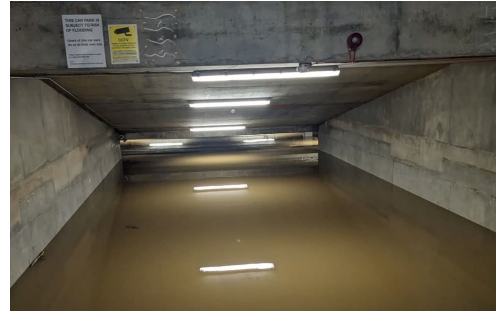
Flooded sloped entrance to underground carpark, Candleford Court, Buckingham
