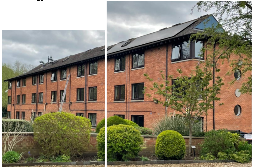
Beloff House from Tanlaw Mill (applicant's photos) Existing roof on left, Proposed roof on right
