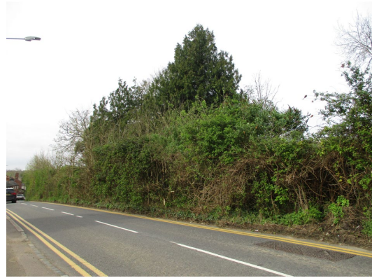
The verge south of the access where the new retaining wall is proposed
