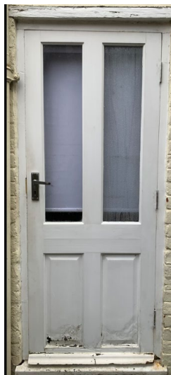
The existing door and the damage
