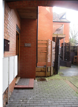
View from arched passage of remains of courtyard with entrance to existing flats A, B & C on left. A new window is proposed in the brick wall
