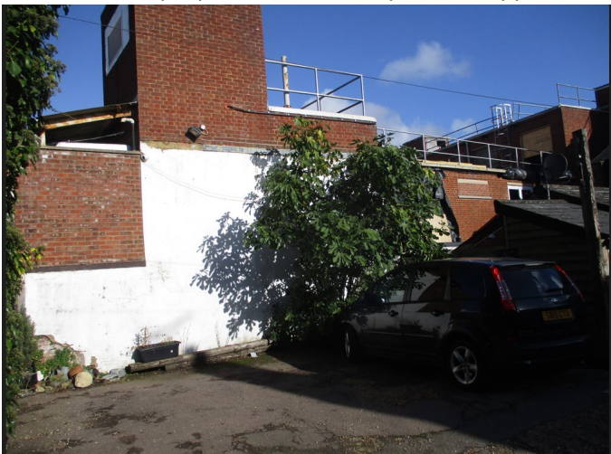
The south side wall from the Forge Cottage access. (taken 26/10/23 for the previous application)
