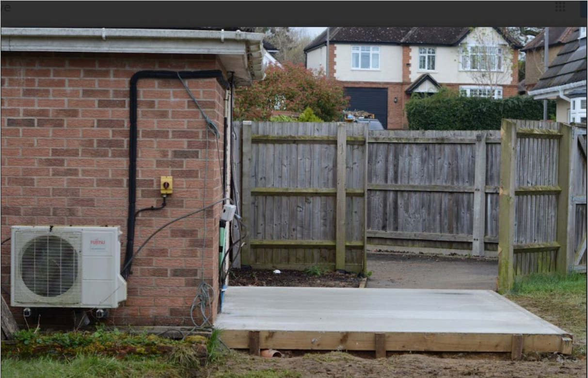
Neighbour's photo of shed/porch slab, drainage pipe ↑ and wiring during construction (April 2023)
