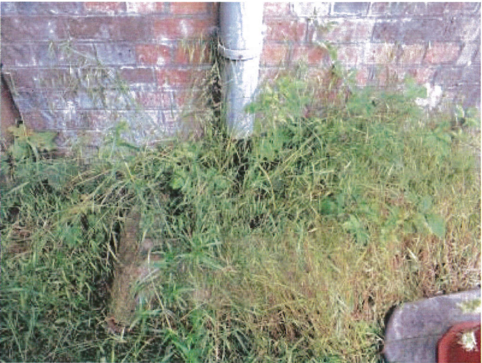
Photo 10: Overgrown vegetation in gully at drain on south face of pier 2/3
