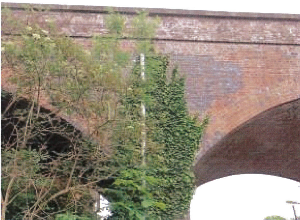
Photo 12: Ivy growth on spandrel wall above pier 3/4 on north elevation.
