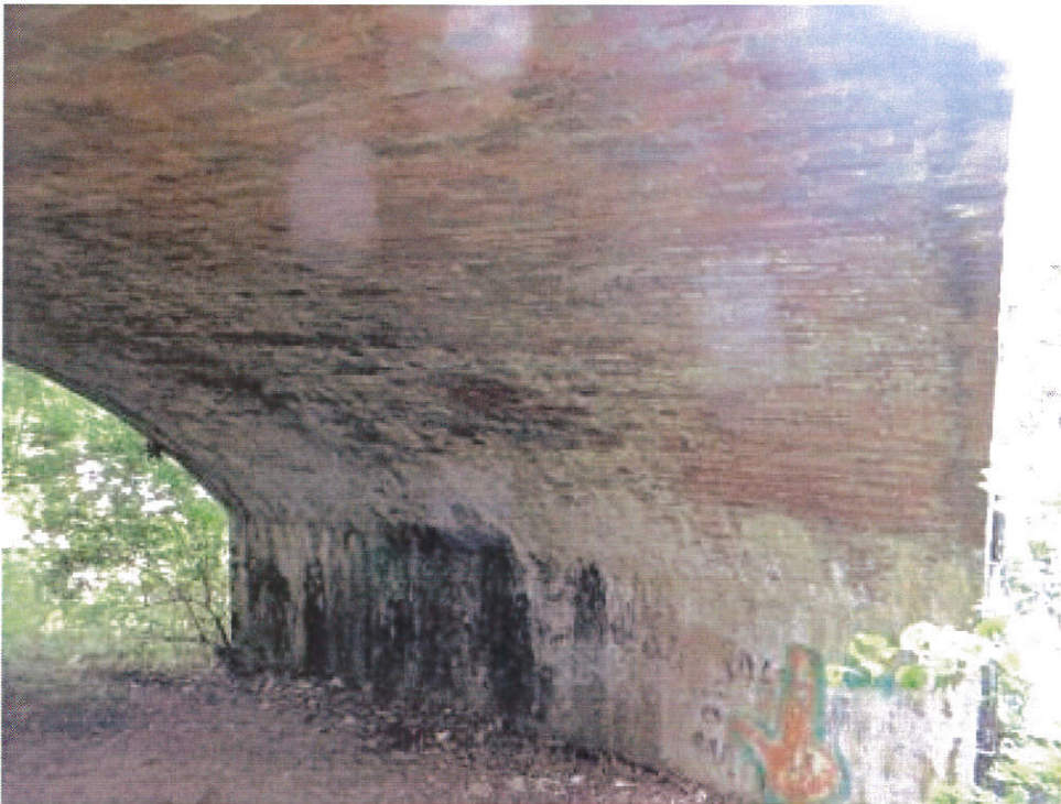
Photo 5: Span 1 arch soffit leachate staining
