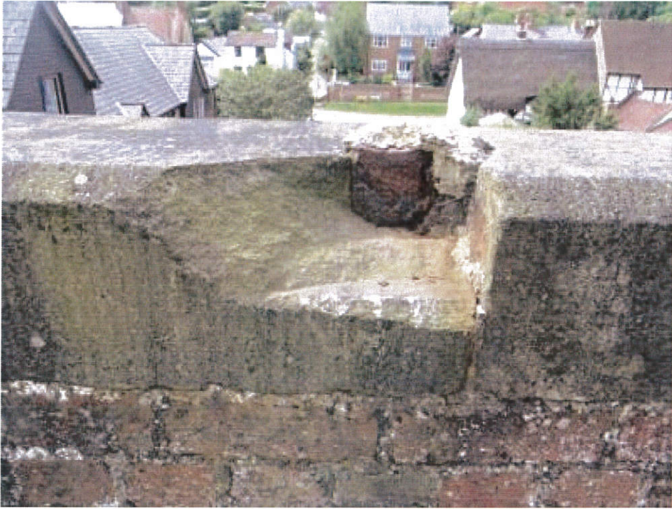
Photo 17: Spalling to coping stones.
