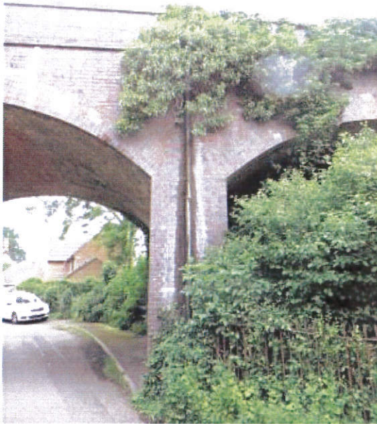
Photo 13: South elevation of east pier. Water leakage on brick face.
