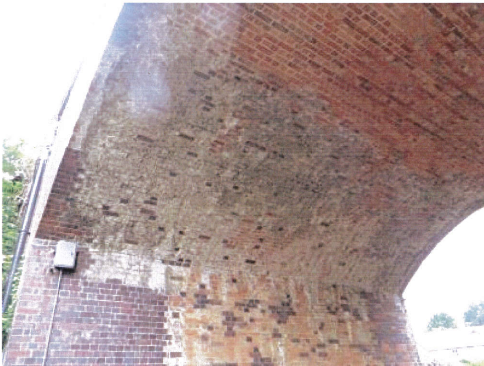
Photo 6: West side of Span 2 soffit with staining.
