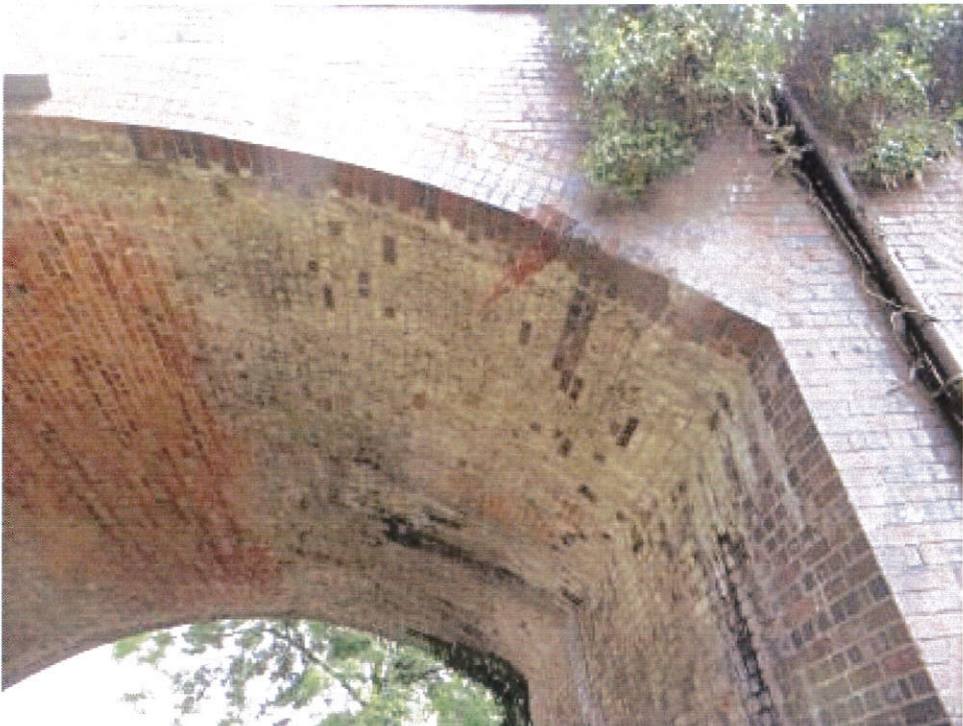
Photo 7: East half of span 2 arch soffit with impact damage on south elevation.
