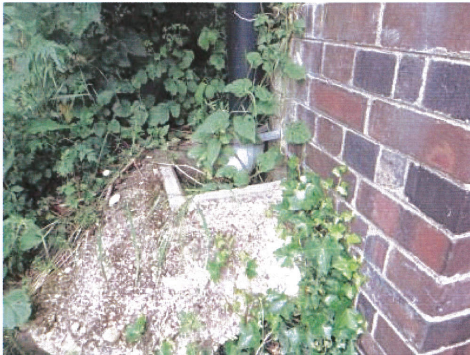
Photo 12: Gully at base of drain pipe on north elevation of east pier.
