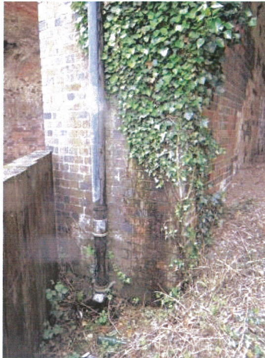
Photo 11: North elevation of west pier. Water leakage on brick face.
