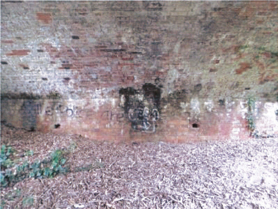
Photo 8: Abutment at span 3 with missing bricks.
