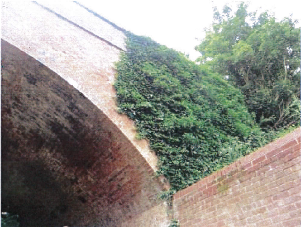
Photo 14: Ivy growth on spandrel wall at east end of south elevation.
