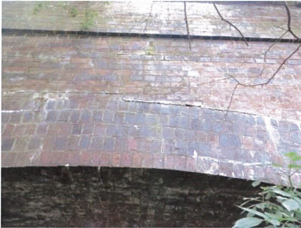
Photo 7: Span 1 North Spandrel – Crack above arch barrel
