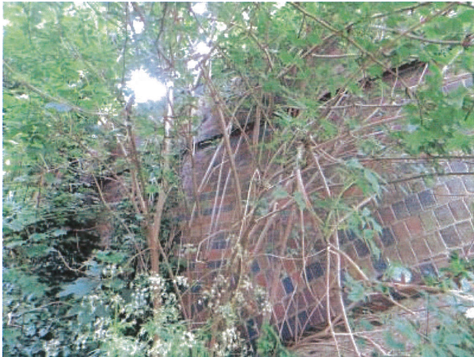
Photo 10: North east corner of span 3 with adjacent small tree growth.
