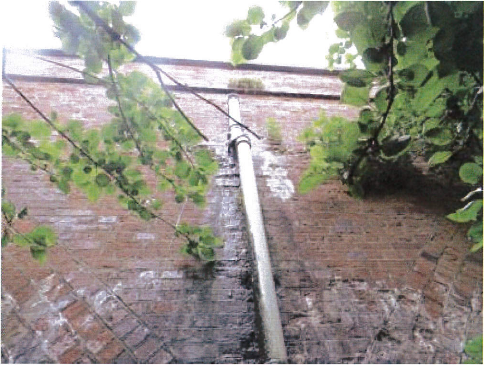
Photo 9: Misaligned drainage pipe on south elevation aboe pier 1/2
