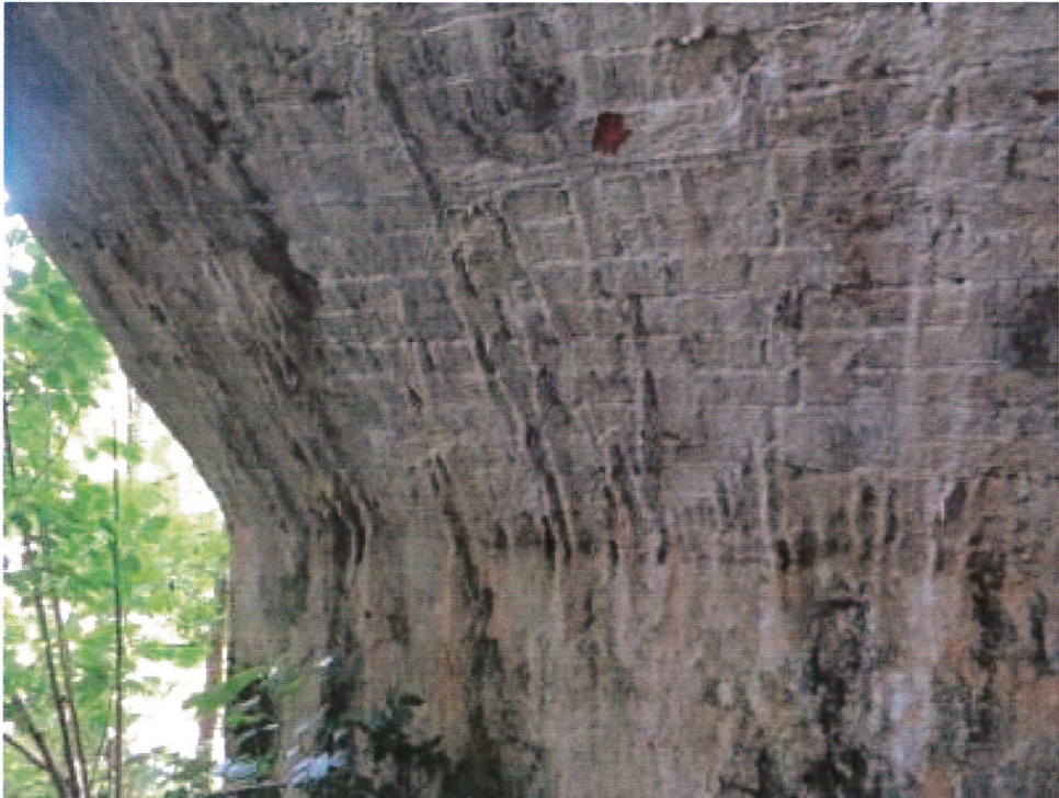
Photo 6: Span 1 arch – heavy leachate build up.
