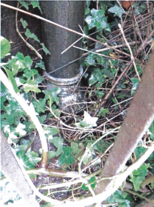
Photo 14: Gully at base of drain pipe on south elevation of east pier.
