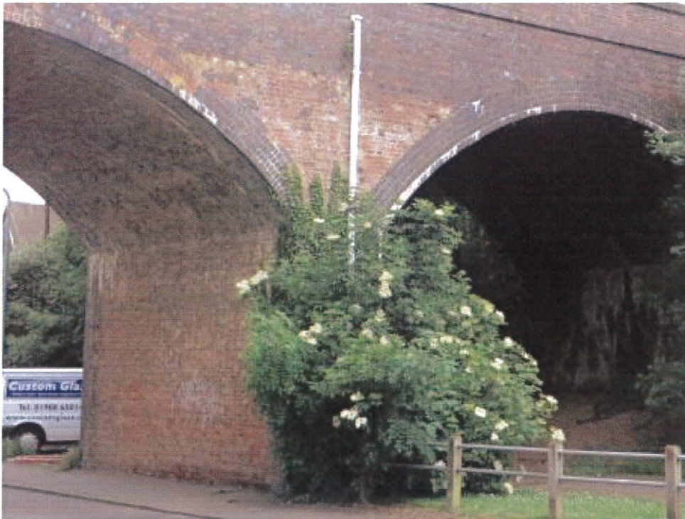
Photo 11: Overgrown vegetation at north elevation of pier 2/3.
