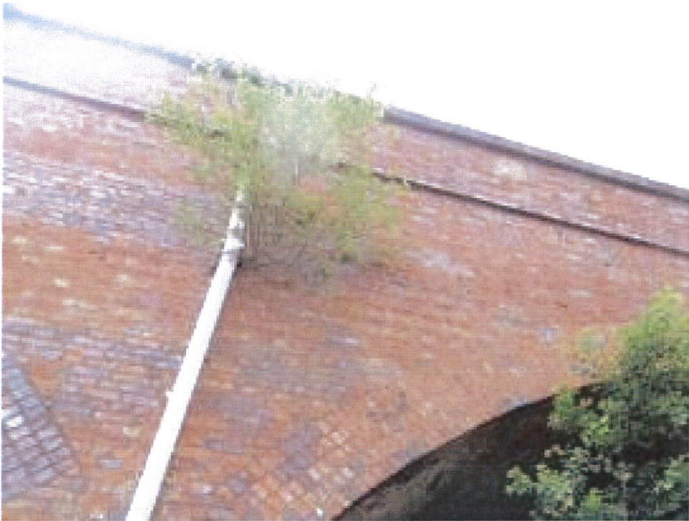
Photo 13: Established plant growth above pier 3/4 on south elevation.
