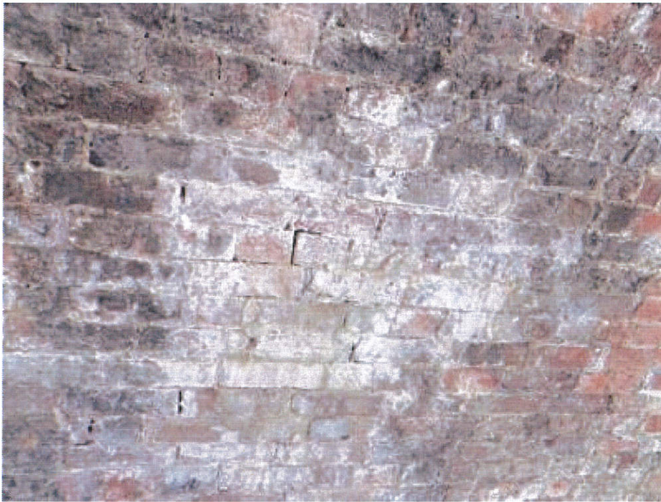
Photo 9: Small area of pointing loss on span 3 arch soffit.
