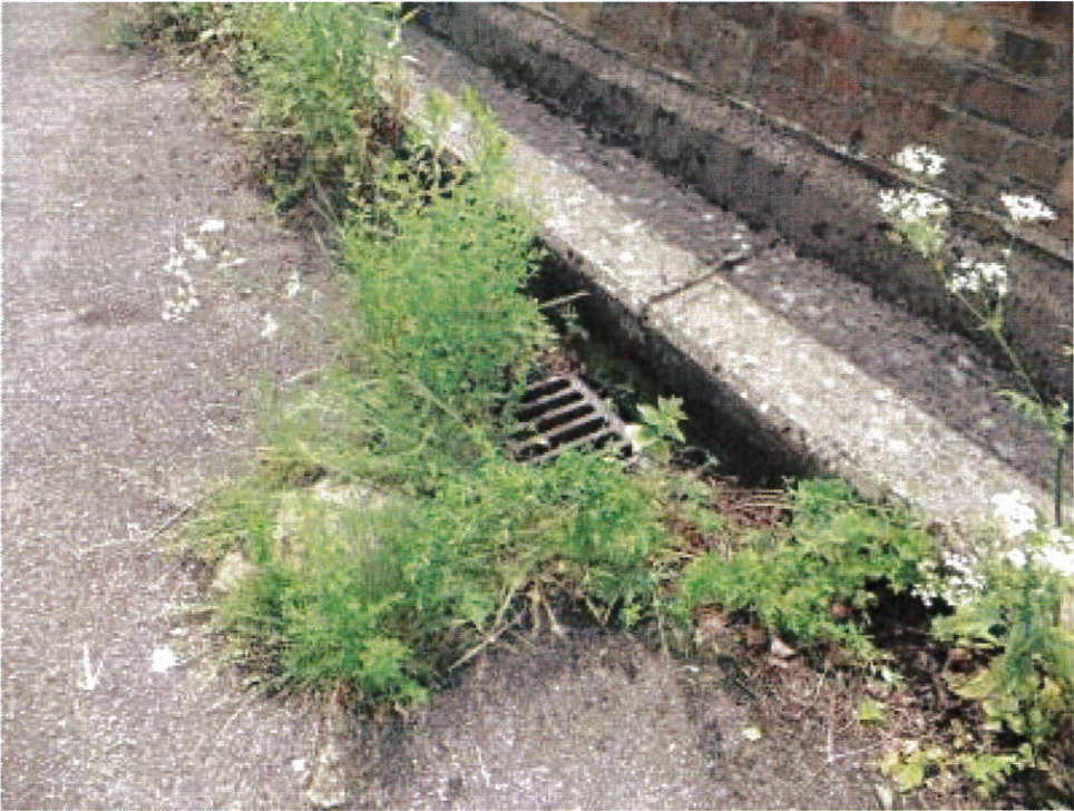
Photo 16: Vegetation growth around drainage gully at upper level.
