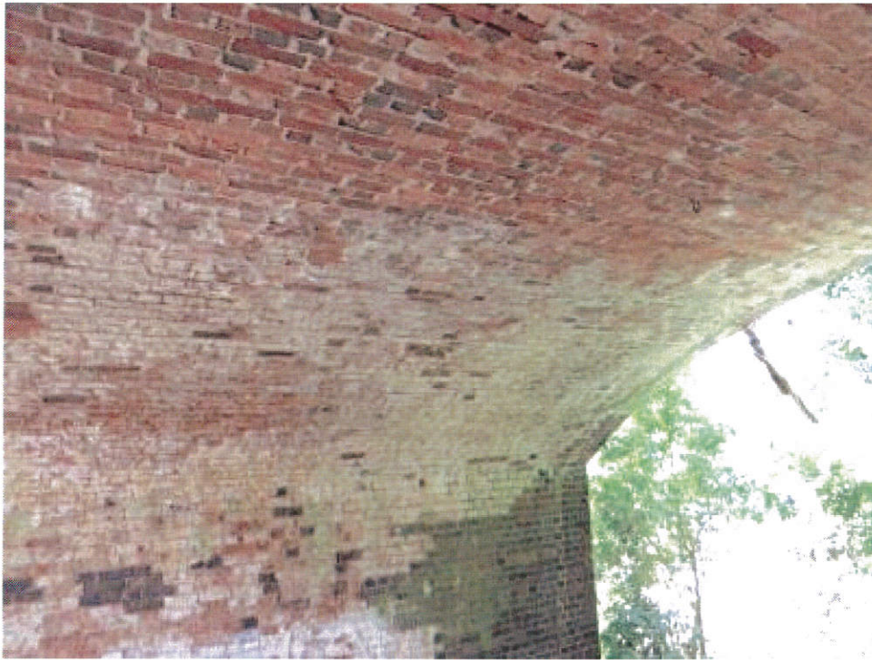
Photo 5: Span 1 arch soffit with staining.
