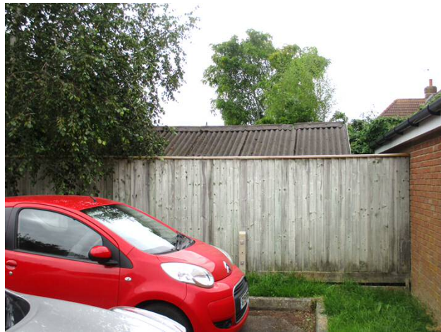
Separation between existing shed and rear wall of garage
