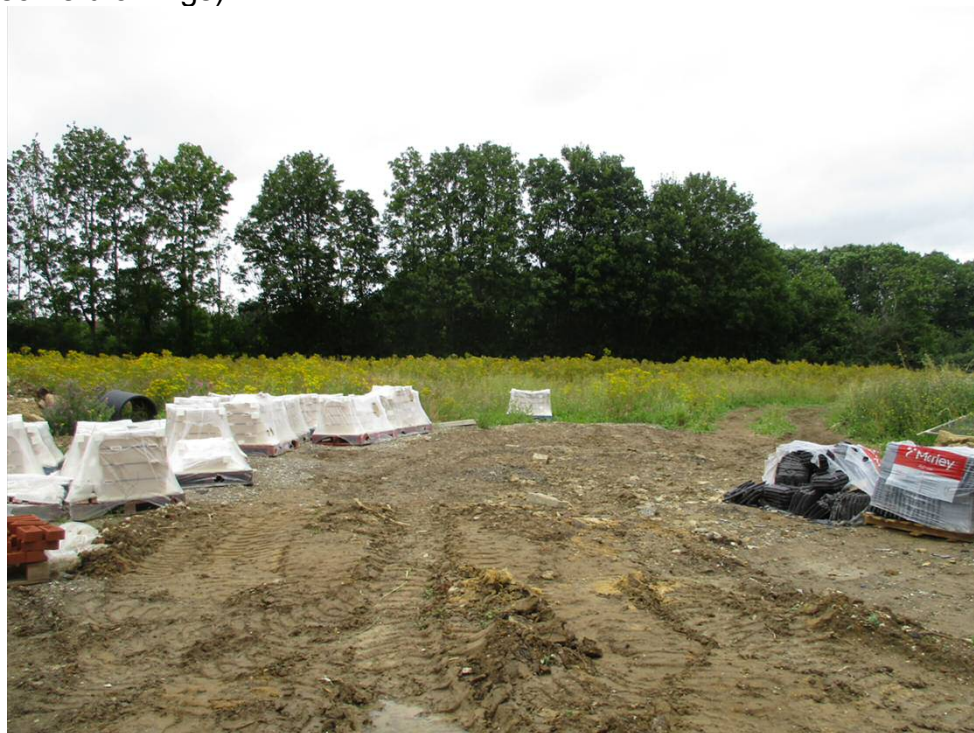
Photo taken from access road beside the substation, ie approximately at the fork in front of the building in the site plan drawings, and looking towards the bypass. The building materials are for the Care Home under construction to the east. Taken 13/8/21
