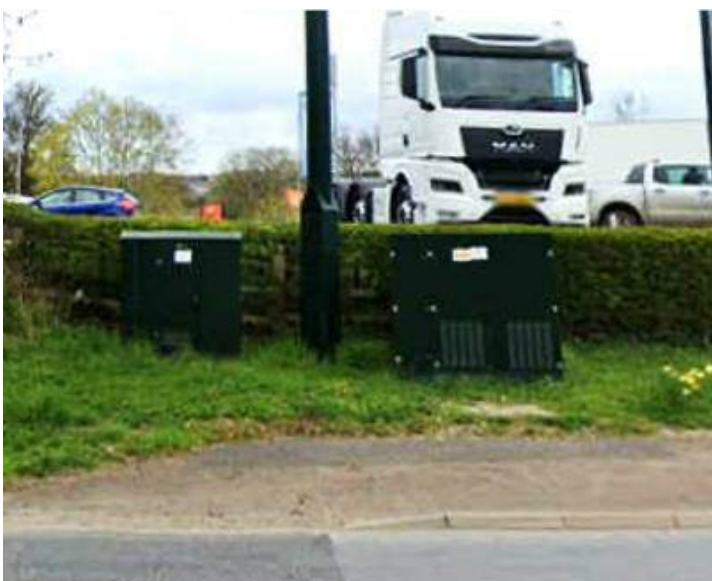
The existing cabinets
