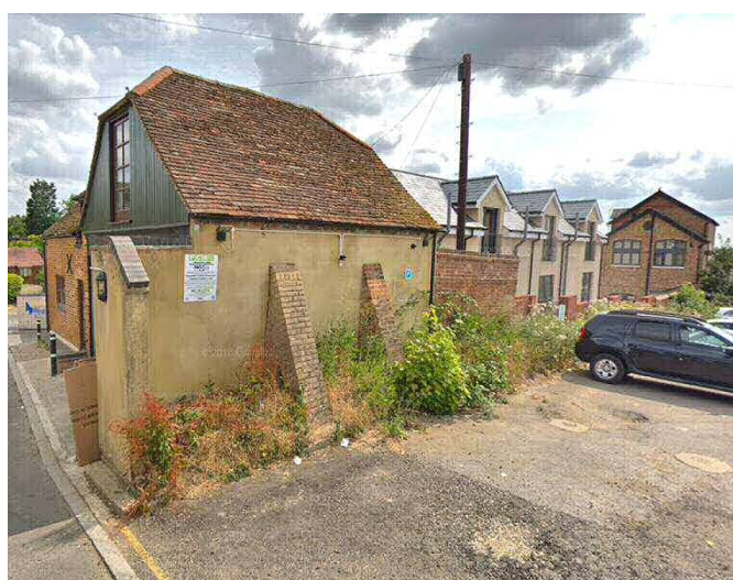
The West wall has already been braced, buttressed and rendered. Adjacent buildings are 23/23A/23B Moreton Road (centre) and Buckingham Lofts (right). The treatment of the historic wall forming the boundary between these buildings and the foreground car park is a matter for on-going discussion between the HBO and the applicant with a retrospective application to turn the three houses into six flats (18/01098/APP; as yet undecided)
