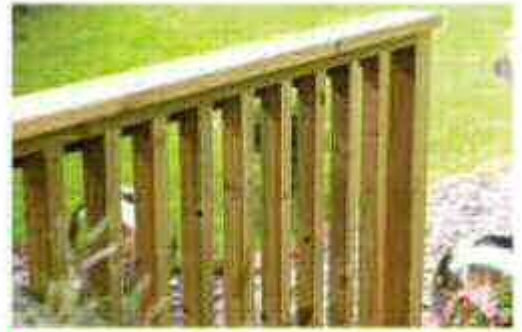
3,4 Decking balustrade near trees
